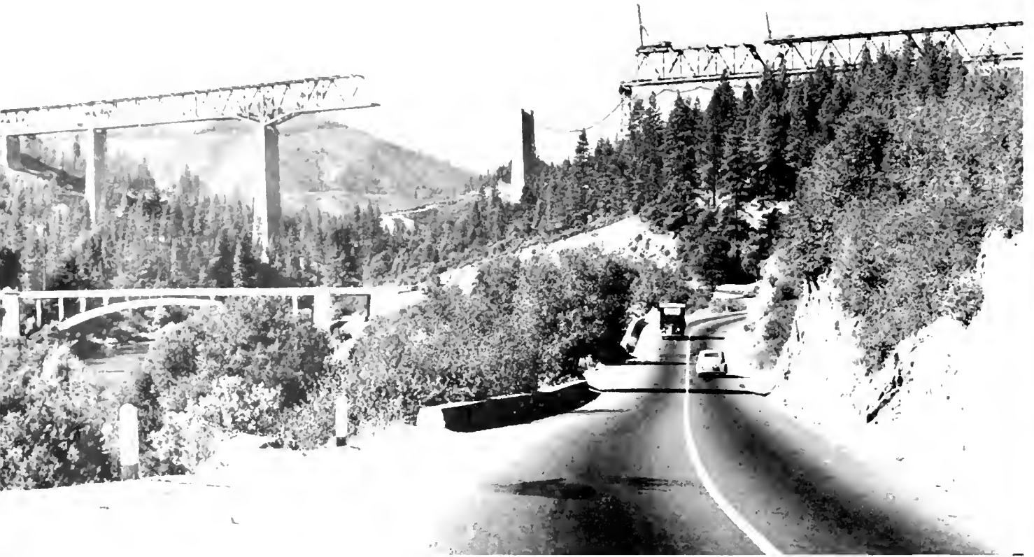
Pit River Bridge as seen today from U. S. 99 with the gap half closed between the great central piers and only another half span to be completed. In the foreground is the existing concrete bridge that will be submerged 335 feet under water
